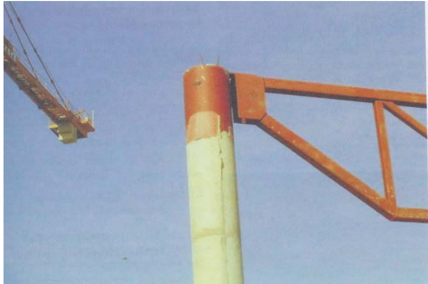
Figura 4. Detalle cabeza pilar con collarín. Figure 4. Detail of union between column and roof structure.
