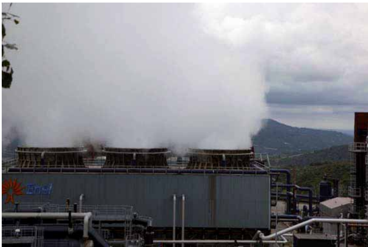
Fig. 6.2. Geothermal Power Plant Bagnore 3. Photo by the author
