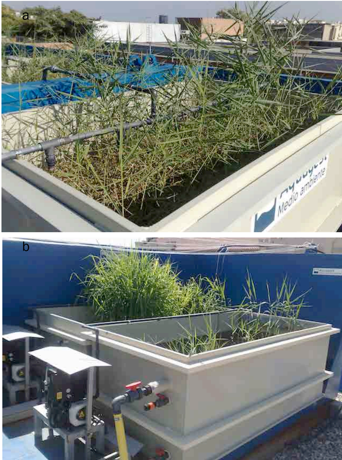
Figure 5.3. View of the vertical subsurface flow constructed wetlands and their distribution pipes (a); horizontal subsurface flow and free water surface wetlands (b) in the experimental hybrid constructed wetland system located in Barcelona.
