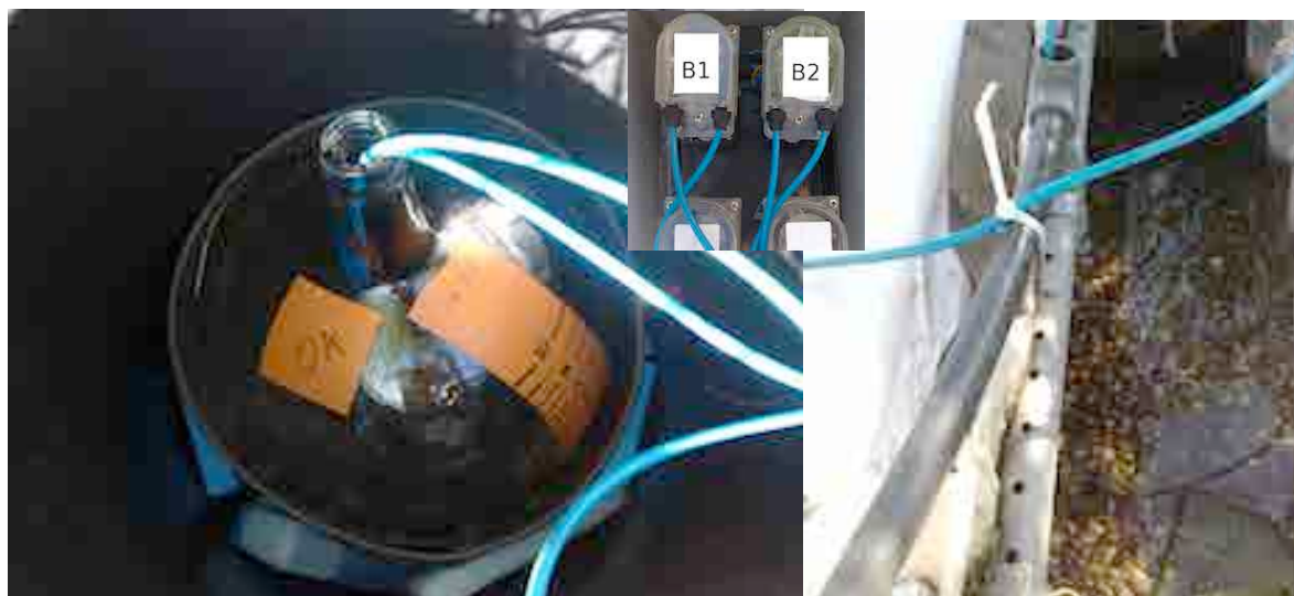
Figure 3.2. View of the doped solution, which was not exposed to light (left), the peristaltic pumps (center) and the injection wires which delivered the solution in the inlet pipe of the horizontal subsurface flow constructed wetlands (right).
