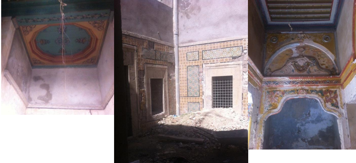
Figure V-2 Current unfavorable state of some houses in Medina, Dar 'Bou Achour' as example
