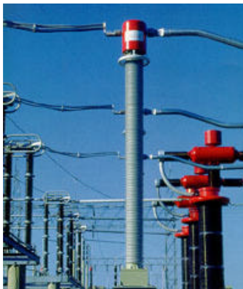
Figure 1.20. 525 kV Optical combined metering unit installed at Bonneville Power Administration - Keeler substation [USA]. Courtesy of Alstom.
