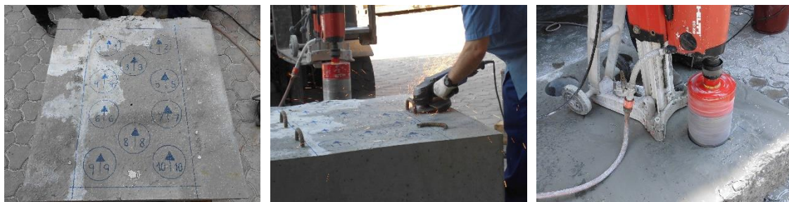
Figure 5.8 a) Position of the cores, b) removal of hooks and c) drilling of cores.
