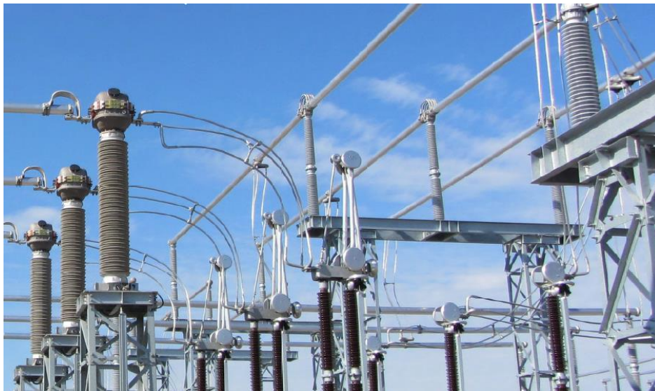
Figure 1-2. Part of an Electrical Substation. Source: SBI catalogue.
