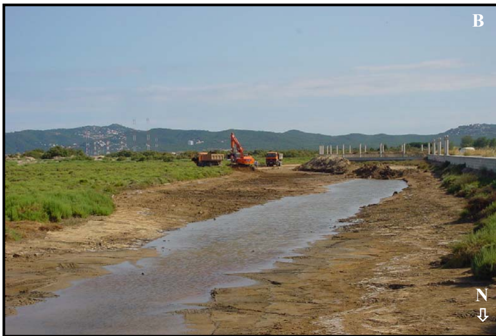
Photo 5. A) Construction of one of the new lagoons (N2) in La Pletera salt marshes. B) The N2 lagoon after its construction. (Photos by Servei de Control de Mosquits de la Badia de Roses i el Baix Ter).
