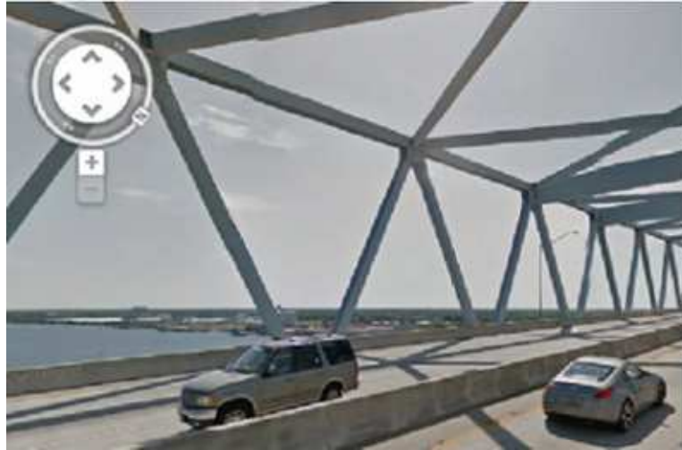
Figure 4.25: Warren truss bridge over Cooper River in Charleston - South Carolina (Source: Google Maps).
