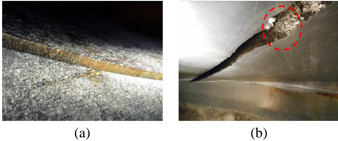
Figure 4-3. Detail of the crack. (a) From the pressure side. (b) From the suction side.
