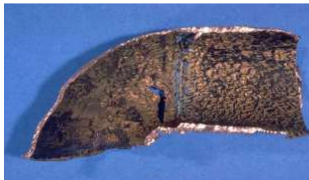
Figure 15. Corrosion-Erosion damage over copper pipe [71]
