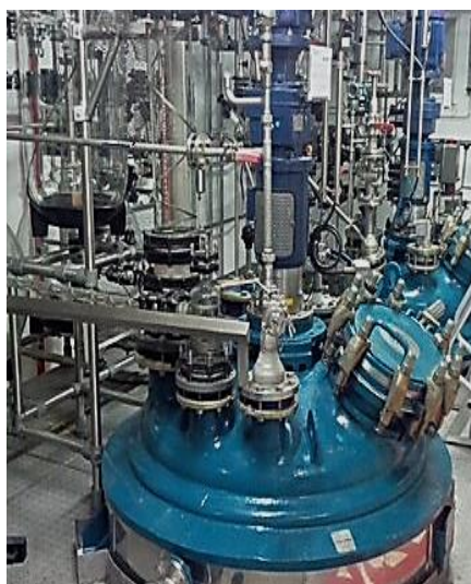
Figure 11. Industrial scale reactor set-up formed by the reaction vessel and multiple pipes and connections required for its operation.
