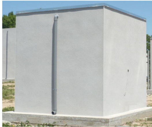
(a) Reference cubicle.
