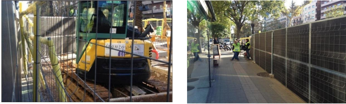
(a) (b) Fig. 3.1: On-site noise control barriers. (a) Construction site area. (b) Sidewalk and neighboring buildings.
