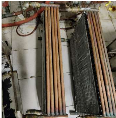
Figure 1.10: Air-cooled condensers in [20]
