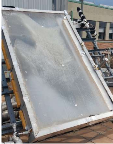
Figure 7.5: A burnt solar collector with TIM inside
