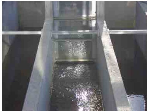
FIGURE 2.11: Sluice gate in the UPC-PAC
