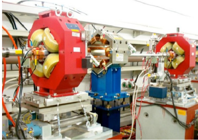
Figure 41: Picture of the installed skew sextupole magnet (SK1) between the QF5BFF (left) and QD6FF (right) quadrupole magnets (red) (Picture courtesy of N. Terunuma).
