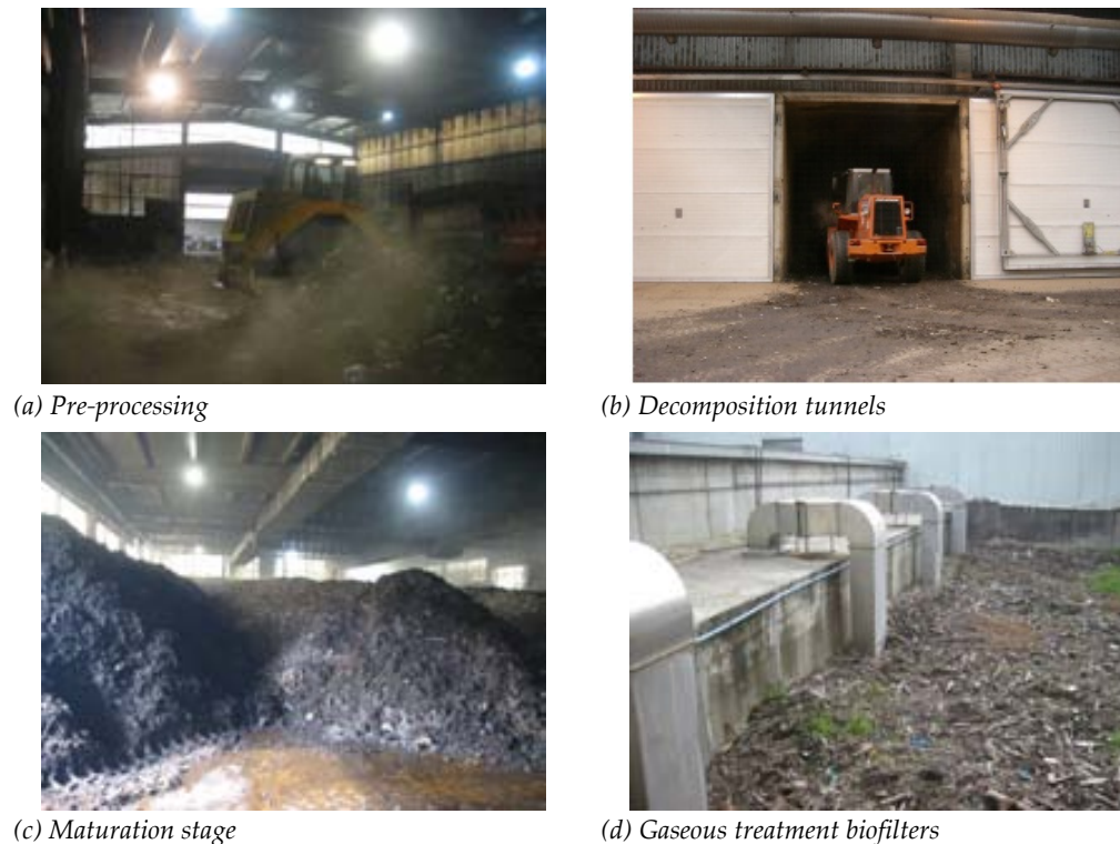
Figure 2.8. Four stages at the industrial composting plant (Castelldefels, Catalonia).
