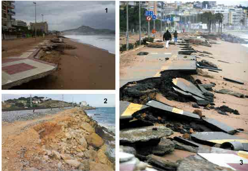
Figure 4.12: Examples of damages caused by storm-induced erosion in the Catalan coast (Location, date and image property). 1: Blanes promenade (La Selva), 2008, LIM; 2: Cubelles (Garraf), June 2009, La Vanguardia newspaper; 3: Blanes (La Selva), December 2008, La Vanguardia newspaper.
