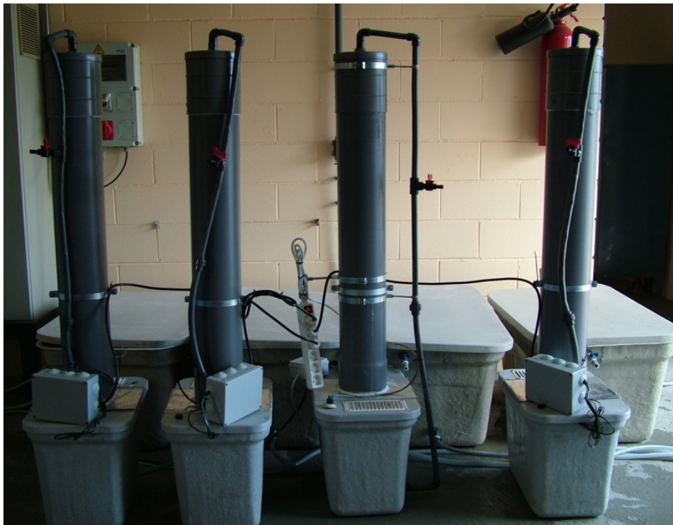
Picture 4.3. Cooling tower demonstrative units located to the Blanes WWTP. The large water reservoirs for each water type are located in the back.
