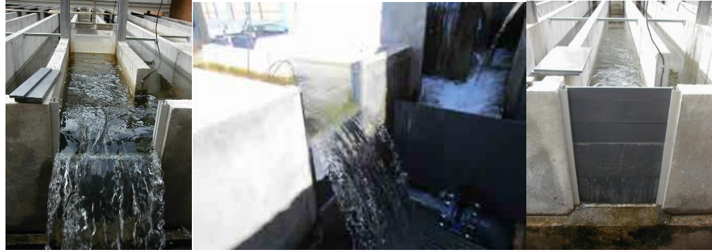
Figure 8.6: Photo of a weir of the canal PAC.
