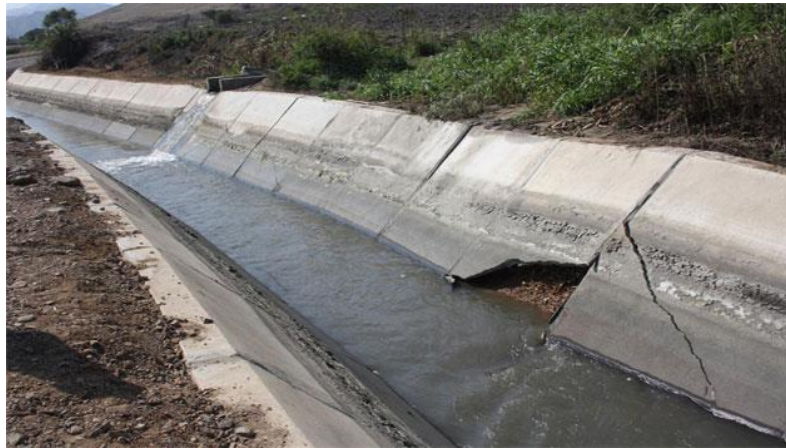
Figure 2.7: Breakage of the cross section of a canal by changes in gradient of pressures (Chimbote canal (Peru)).
