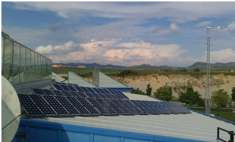
Fig. 2.4. Photovoltaic generator and wind turbine at UPNa
