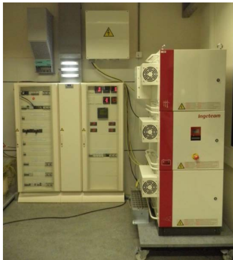
Fig. 2.7. Hybrid power converter INGECON® HYBRID MS30 and switch cabinet which includes the control relays, power analyzers and digital indicators.
