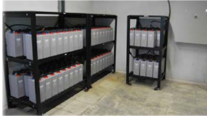
Fig. 2.6. Lead-acid battery bank
