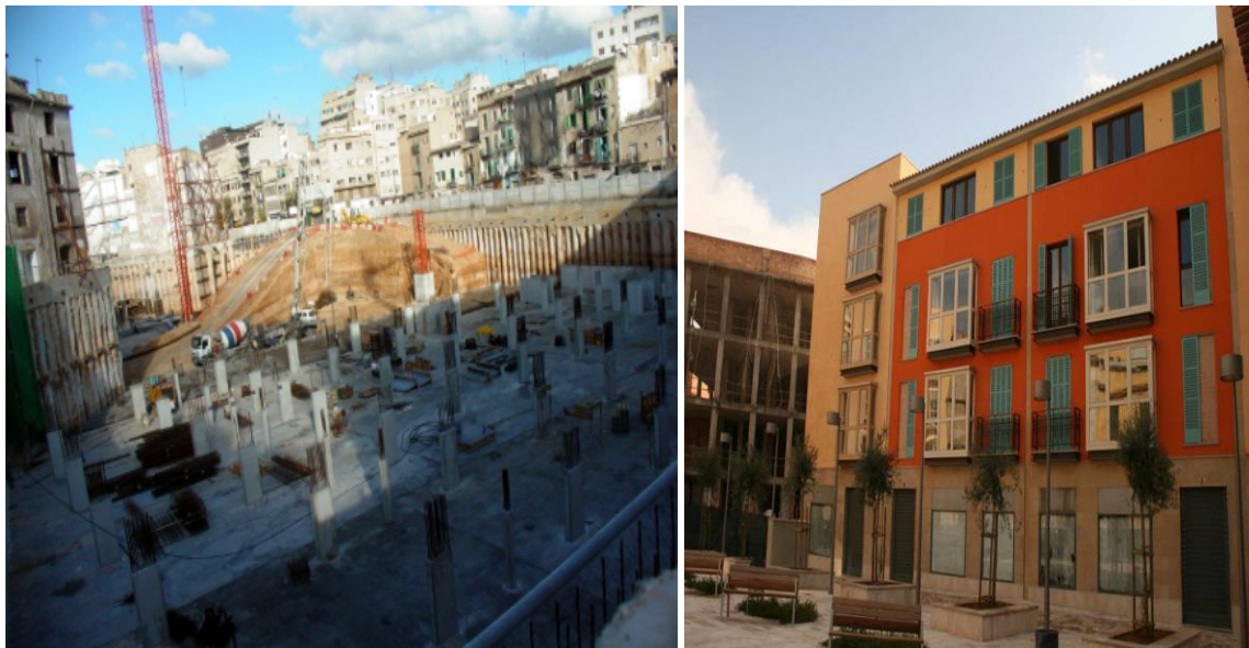
Images 15 and 16: Es Brut soon became Intervention Unit 2B within the overall Special Renewal and Protection Scheme for Es Barri (PEPRI de Sa Gerreria). The photographs show what the site looked like when the underground car park was being built and when the properties went on sale. Image 15: Jaume Franquesa and Marc Morell (2004); Image 16: Marc Morell (2008).
