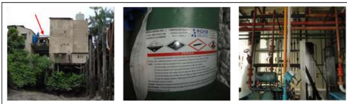
Figure 5.6: Ammonia cylinder employment during the refrigeration process.
