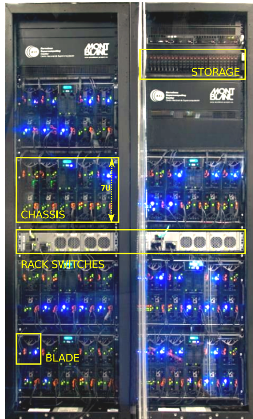
Figure 7.4: The Mont-Blanc prototype: physical view of the entire system.
