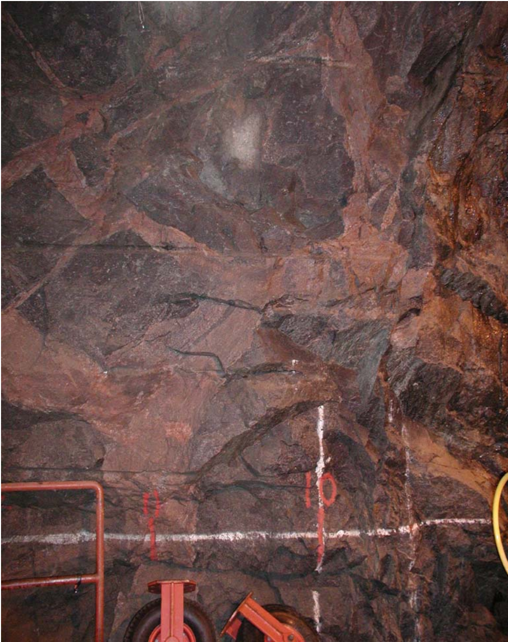
Figure 5.56: Detail of the gallery excavated by blasting closed to the ZEDEX gallery entrance. As water bearing fractures are not present in the area of the picture, the formation seems to be “dry”.
