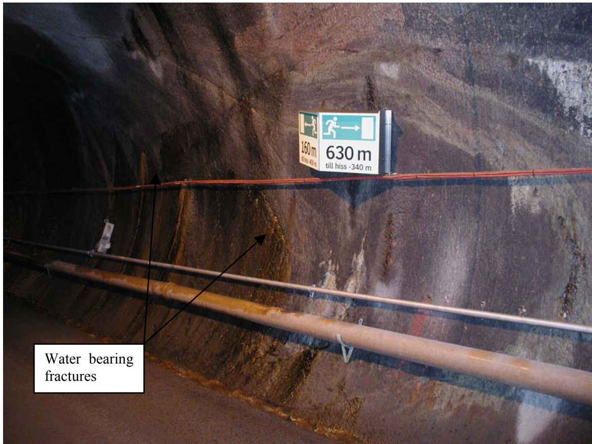
Figure 5.58: Wider view of the main tunnel excavated by TBM. It is also clear that there are water bearing fractures and non-connected fractures.
