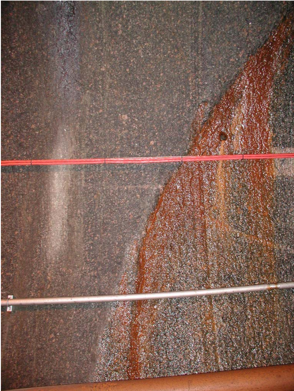
Figure 5.57: Detail of the main gallery excavated by TBM at the third level (-450 m below the ground surface). Water flows through a fracture. Therefore, there is a part where oxidation processes occur and other part where granite seems to be “intact”.
