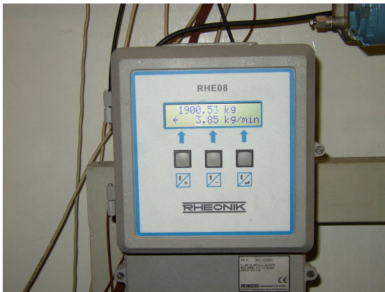
Figure 3.21: Liquid refrigerant mass flow-meter: transmitter
