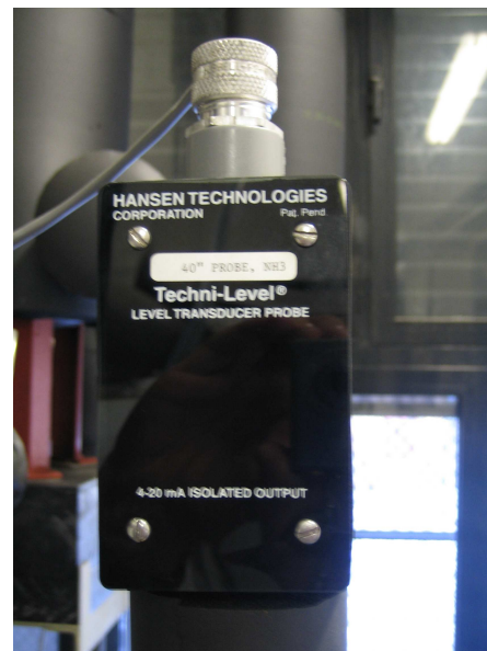
Figure 3.24: Refrigerant liquid level transducer
