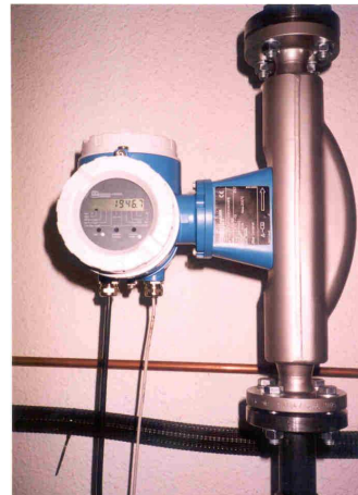
Figure 3.17: Liquid mass flow-meter
