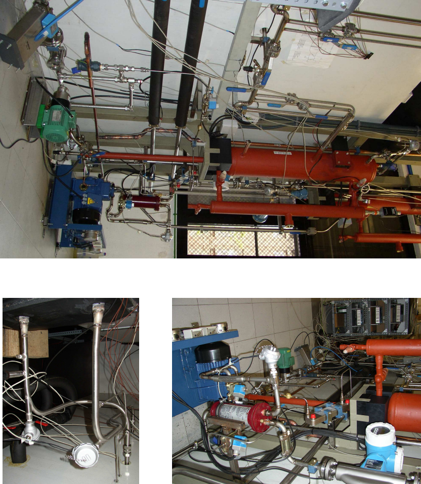
Figure 3.6: Phase-changing refrigerant circuit: Views of the outside circuit with low-pressure receiver, compressor, pump, etc. View of the evaporator connection.
