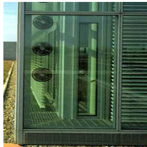
Figure 1.7: Facade with horizontal and vertical ventilation, Gotz headquarters, Wurzburg, Germany. Fans in the corners of the cavity switch on to redistribute the warm air from the sunny to shaded faces of the building.
