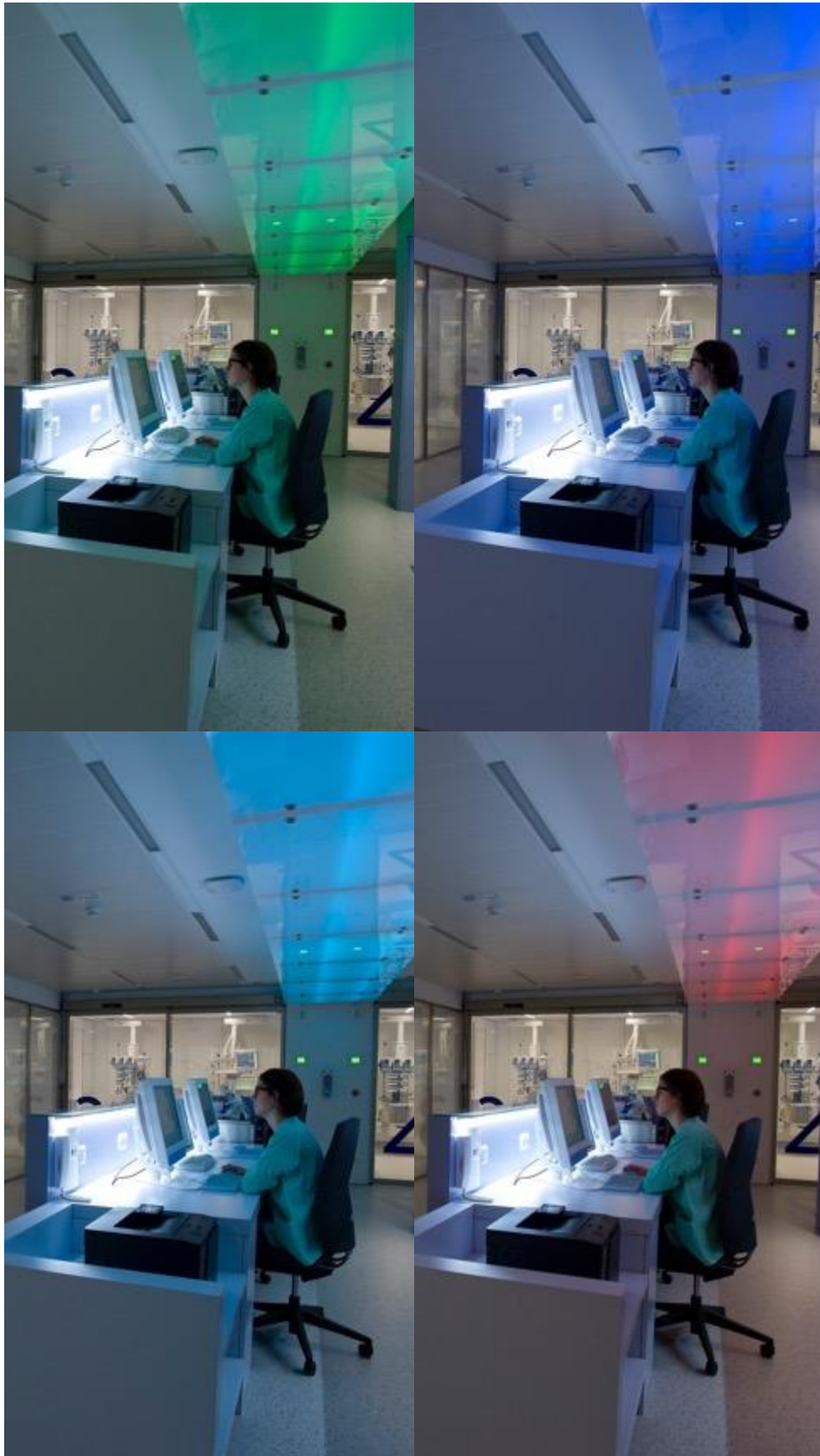
Figure 48. Programming of the Scena Module at the nursing station panel in the ICU.
