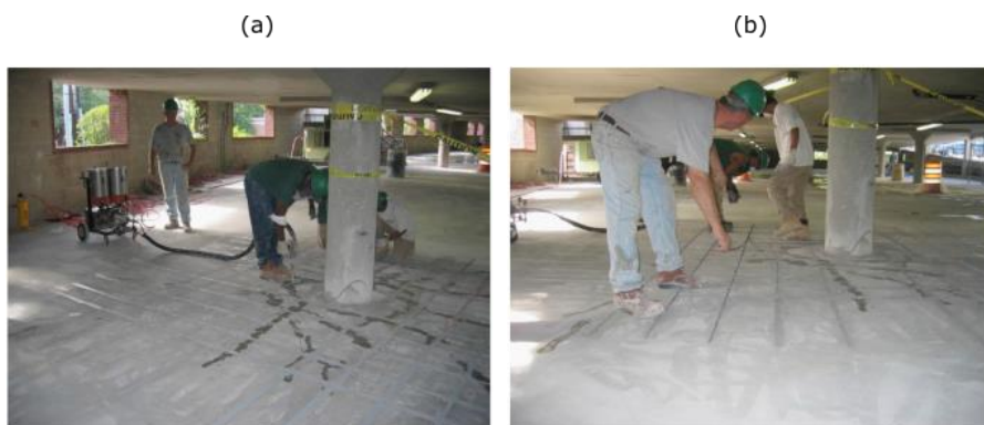
Figure 2.4: Examples of NSM installation: (a) installation of the epoxy adhesive and (b) installation of CFRP bar [17].
