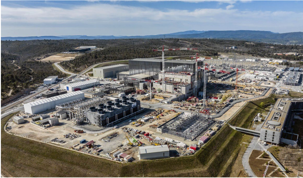
Figure 1.1. Aerial view of ITER construction site in Saint Paul-lès-Durance, southern France (April 14 th , 2022).
