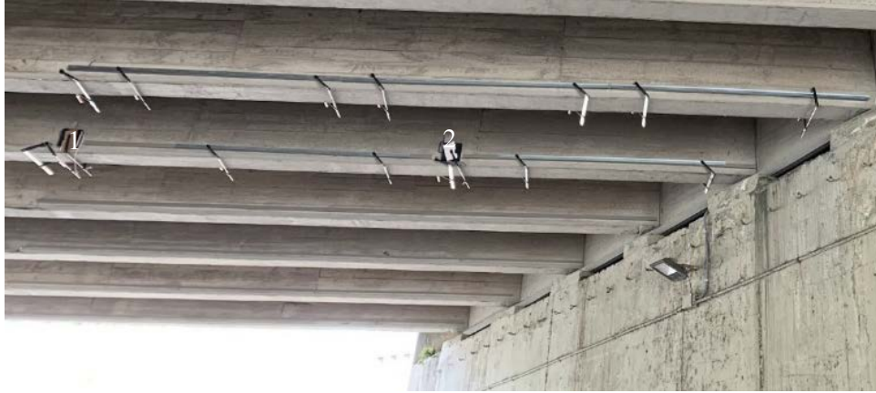
Figure 6-18. Instrumentation of Andoain bridge using two LARA (sensing part only) mounted next to the PCB 607A61 accelerometers.
