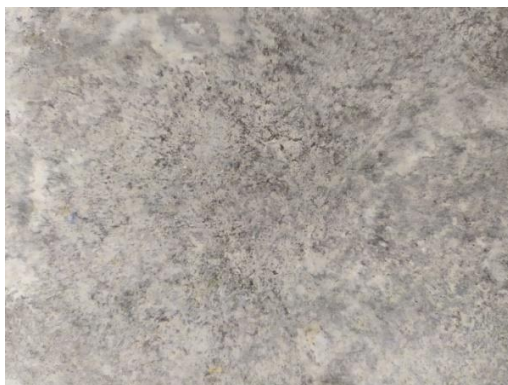
Figure 3-5. Corroded surface after being exposed to the AcOH gas phase for three months, and into the air for approximately one week.
