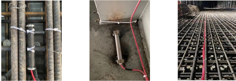
Figure 12. Installation of the vibrating strain meters in the steel and reinforcing bars
