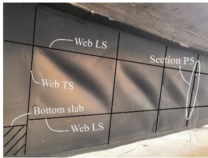
(a) Web buckling in short span
