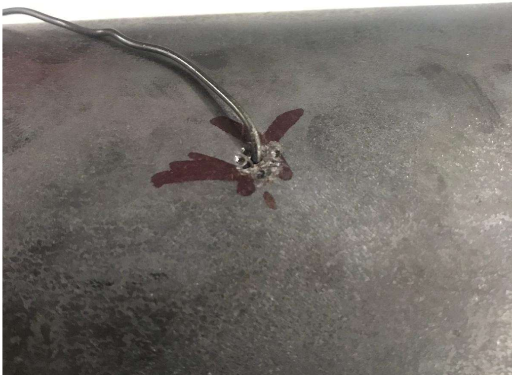
Figure 3-10. K-type thermocouple inside the pipe wall.
