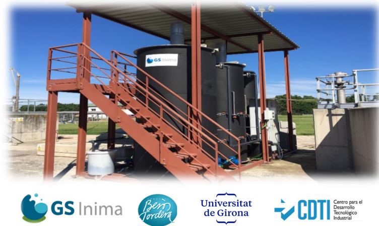
Figure 3.2 Pilot plant 30 m 3 ·d -1 at WWTP Montornès-Barcelona
