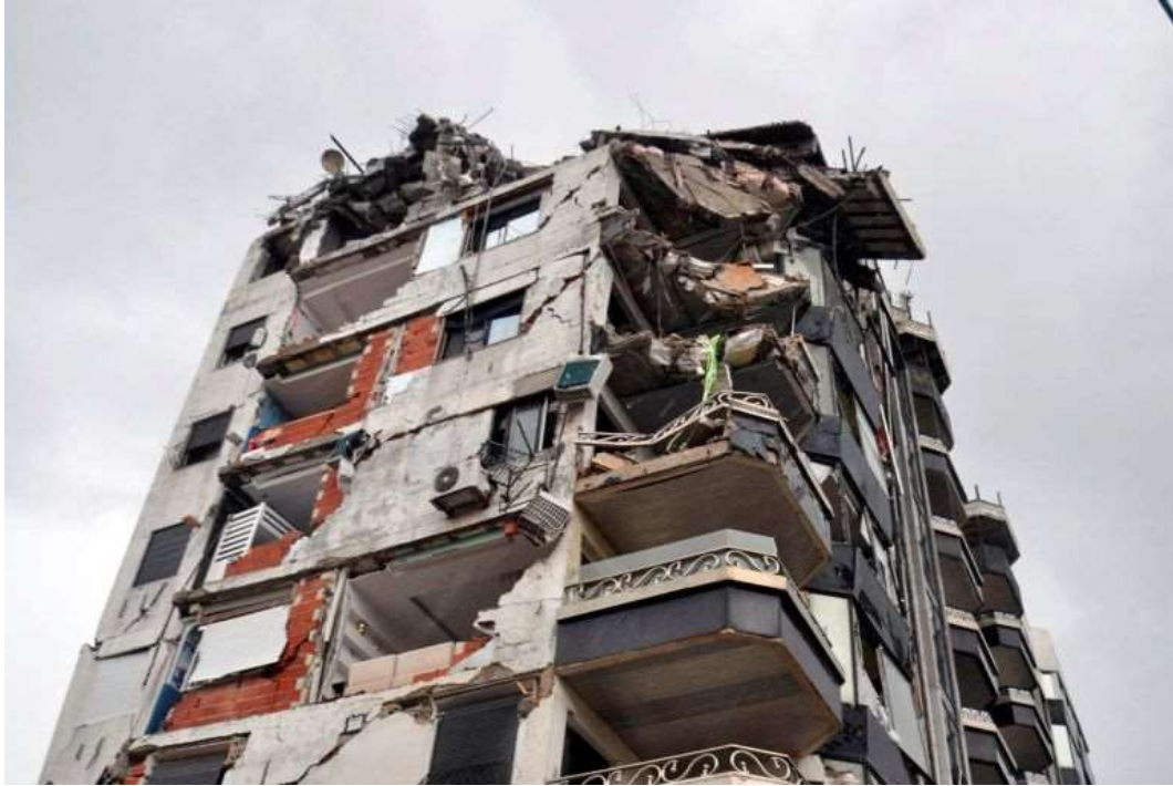
Figure 76 Lattakia City, Jableh, Earthquake (Al-Jazeera Net correspondents, 2023)
