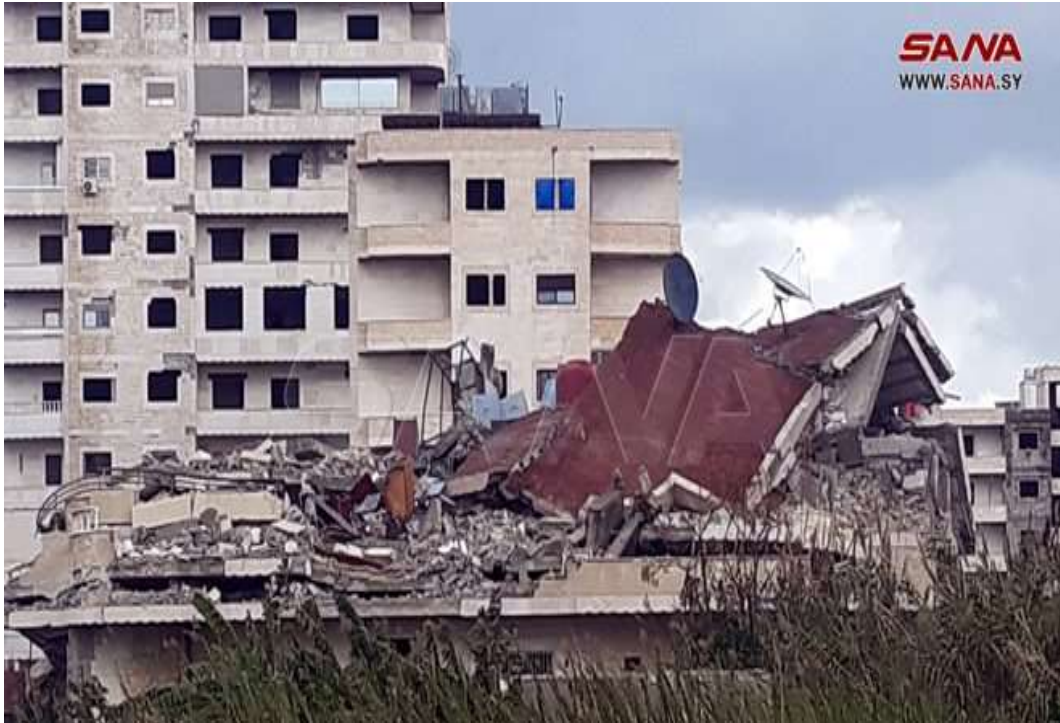
Figure 74 Lattakia City, Jableh, Earthquake (SANA, 2023)
