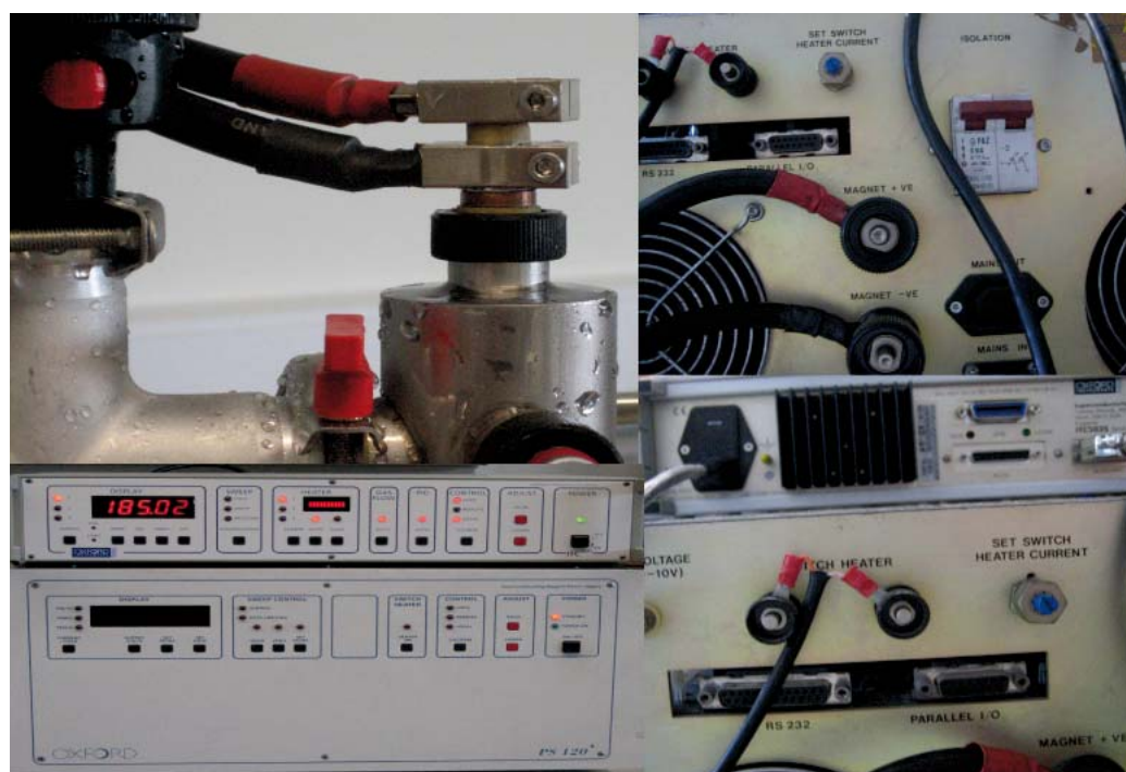
Figure 1.7: Different pictures of the connections between the magnet and the power supply source.
